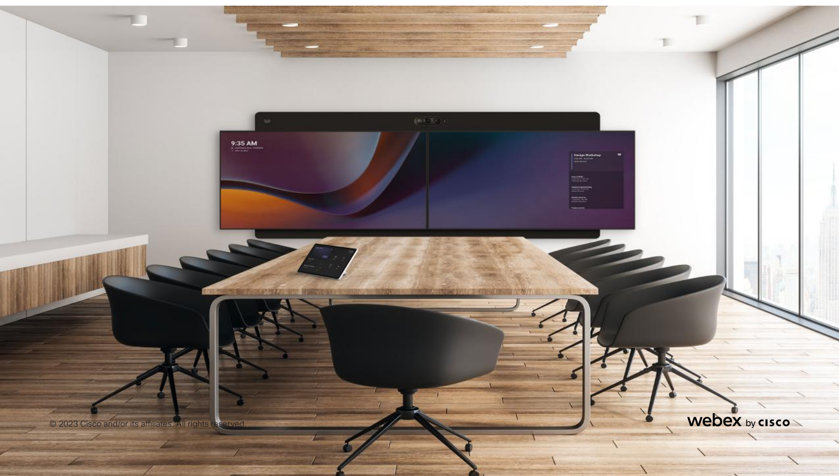
Figure 1. The Cisco Room Kit EQX with wall mount module running the native Microsoft Teams Rooms experience in a conference room.
